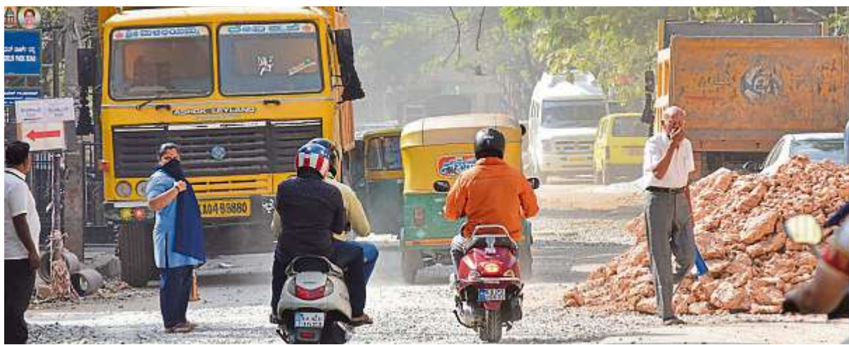
Ongoing road work, unregulated construction and disappearing green cover have contributed to rising pollution levels in the city. (Above) A dug up and dusty road at Seshadripuram. DH PHOTOS BY JANARDHAN B K
